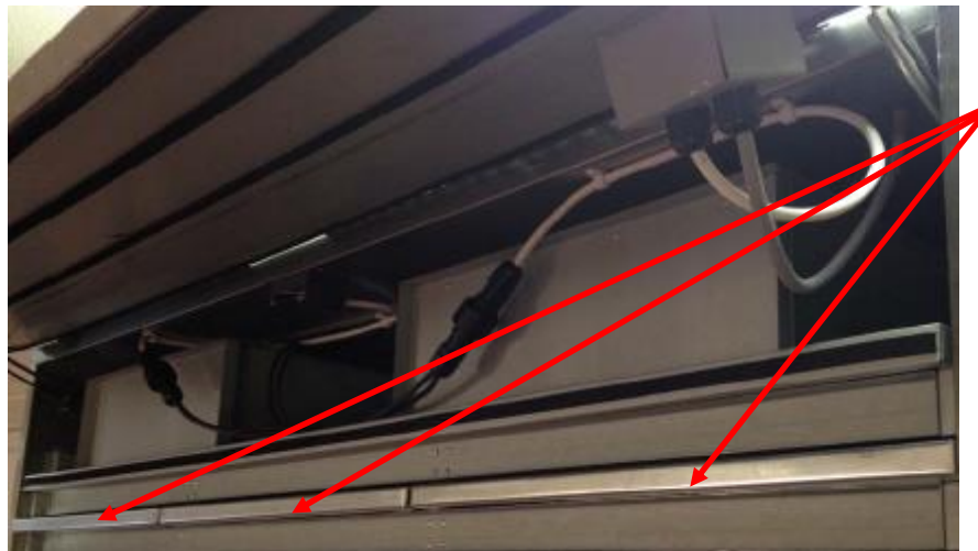
Stage 4 Carbon Filters Behind Access Panel
